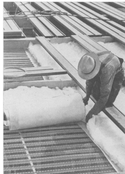
PREVENTING LOSS —Application of glass wool or other insulation prevents loss of what heat you have.
