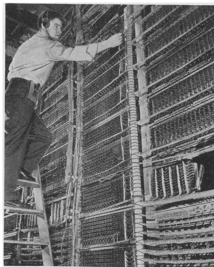
BELL'S BRAINCHILD —An important part of the telephone system, the main switching system at the Bell Telephone Laboratories duplicates every type of switching circuit in use in the telephone system today.
