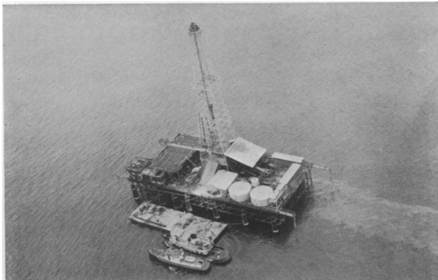
BORING UNDERWATER —Ten miles out in the Gulf of Mexico the search for hidden oil goes on. This picture shows the operation of well-boring underwater from a platform by the Magnolia Petroleum Company.
