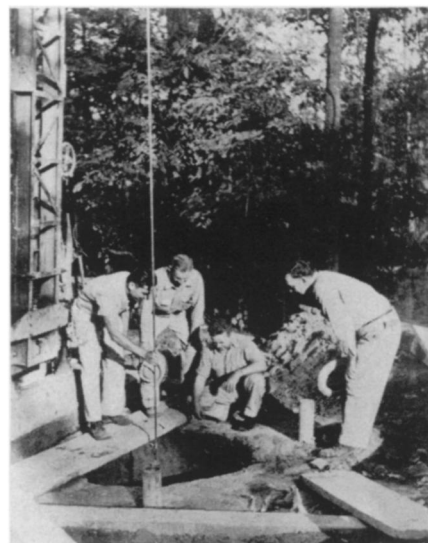
GASIFYING COAL —A large-bore hole is sunk to the coal seam in the second trial at the Alabama underground coal-burning experiment.
