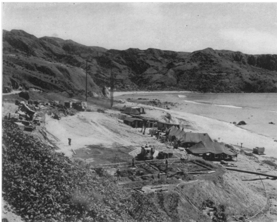
ISLAND LORAN STATIONS —Four more Loran stations have been installed in the Far East area of the Pacific to aid navigation by airplanes and ships. Shown here, in the early stages of construction, is one of them, the new Coast Guard transmitting station on Bataan Island. The stations can transmit their signals over an area of 750 miles by day and 1,400 miles by night.
