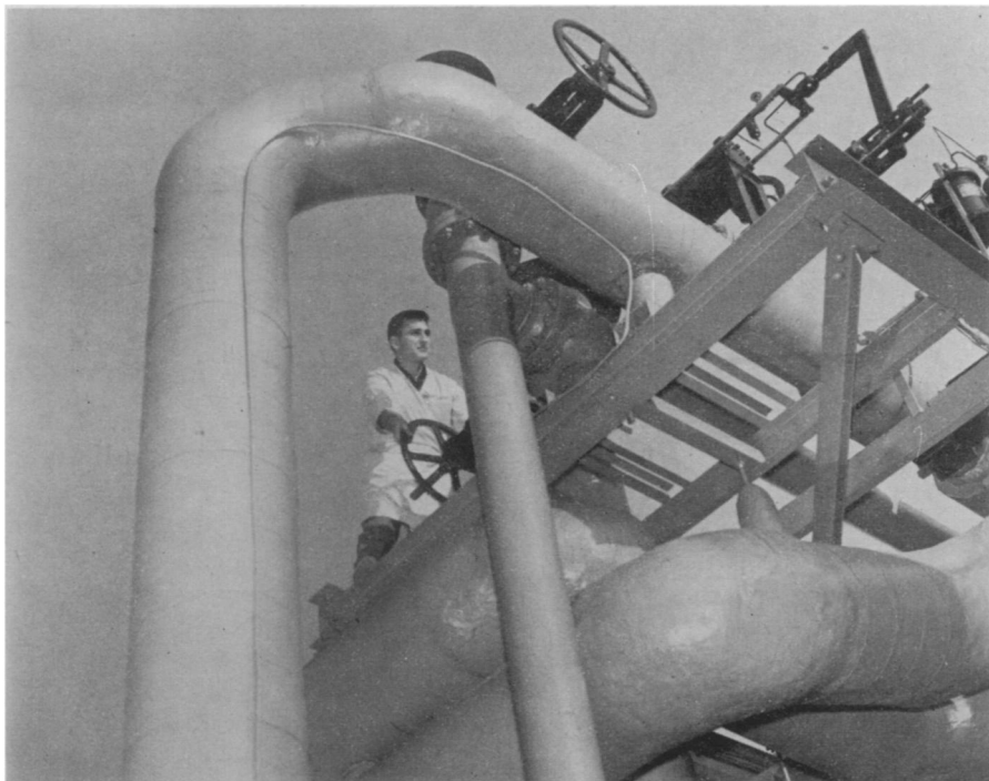
TEST "PILOT" —This network of massive pipes at the new research facility of Bendix Aviation Corporation connects the powerplant with actual test cells where supersonic speeds and high-altitude atmosphere are simulated.
