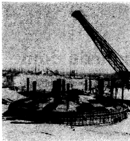
Waste tank: Storage, not disposal.
