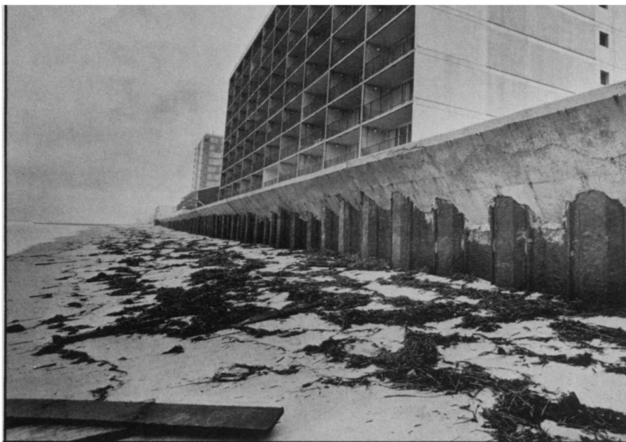
Before a winter storm, sand on Ocean City's beach reached to the top of the seawall.
