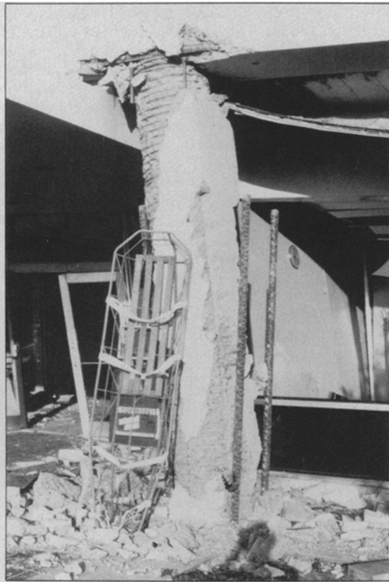
Concrete pillars with vertical steel rods (left) are brittle and may fail in an earthquake. Ductile concrete pillars (right) with additional helical steel windings have proved more durable.
