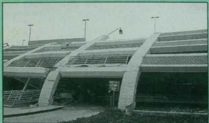
Collapsed parking garage in Northridge.
