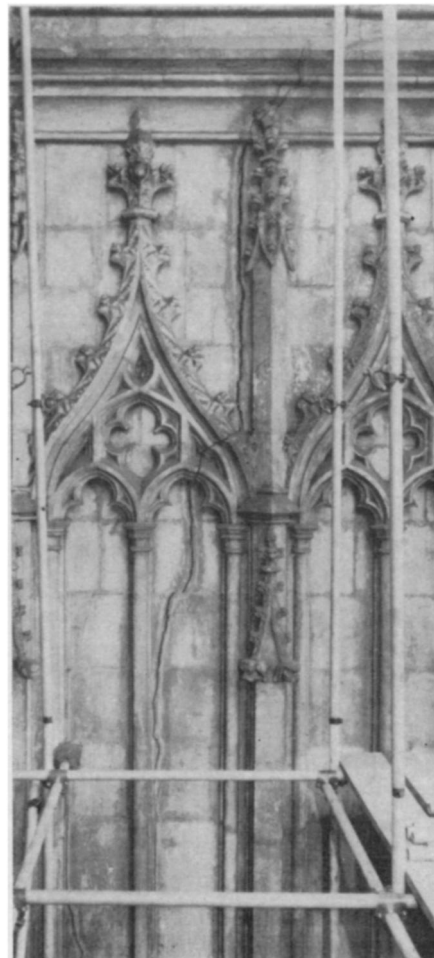
Crack in a tower wall 120 feet up.
