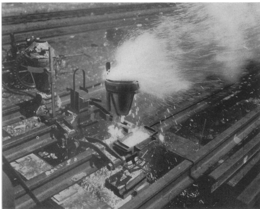
SPEED WELDING —This funnel-shaped crucible spewing thermite fire is welding rails for a quick replacement job.
