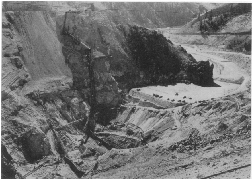
BIG DAM —Conveyor belts play an important part in the building of this huge 444-foot earthen dam for the U. S. Bureau of Reclamation. Impervious clay for the core of the dam is brought from a borrow pit a mile and a half away by nine flights of Goodyear belts. After it is dumped at the site, it is spread in six-inch layers and tamped with sheepsfoot rollers, drawn by Diesel tractors. The earth which will be packed on both sides of the core will be drawn from two other pits. The upstream side of the dam will be reinforced with heavy stones for the dam's entire height.
