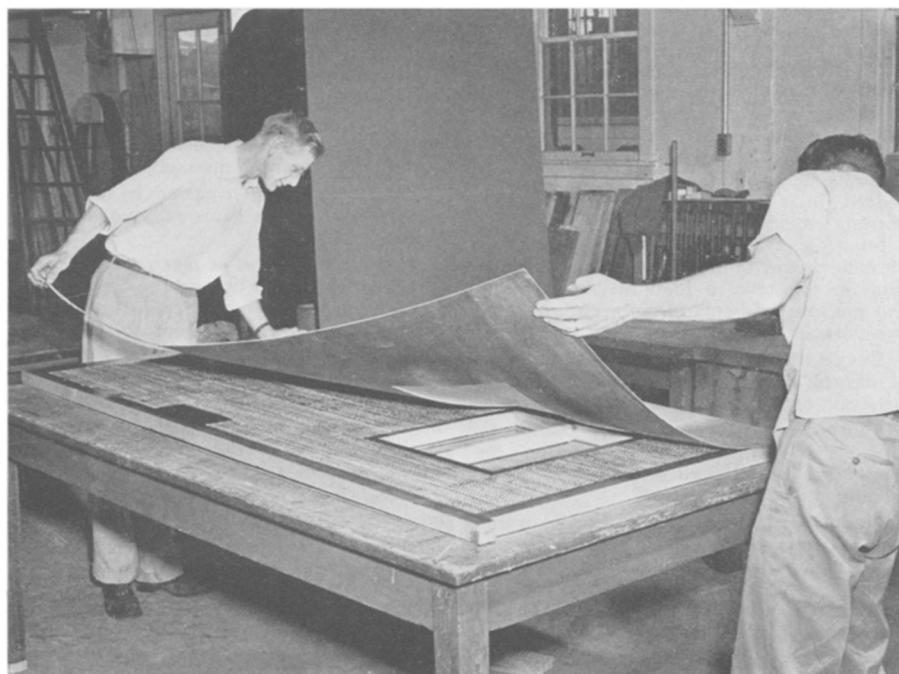
HONEYCOMB SANDWICH —This type of panel construction has gone into the building of an experimental house by the government. The core, which is the insulating material, is shaped by special machinery to resemble honeycomb. The picture shows a plywood cover being placed over it to be bonded to the core by a highly water-resistant phenolic resin glue. (See page 397.)
