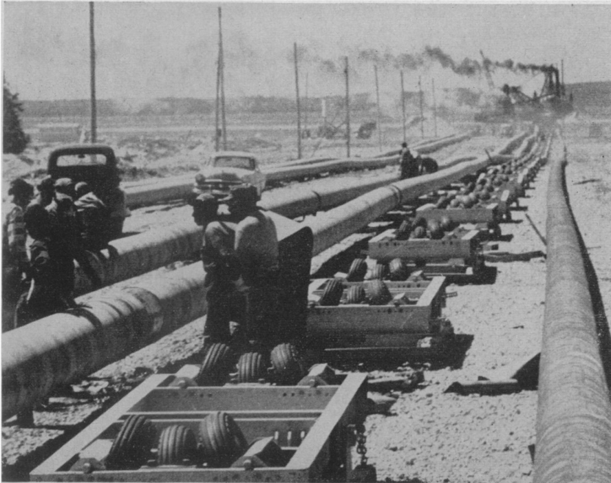
LABOR-SAVING DOLLIES —Rushing to complete the laying of two four-mile sections of 20-inch pipe along the bottom of Mackinac Strait before the winter freeze, contractors saved more than 100 miles of land clearing and ditching by crossing the 240-foot deep shipping channel with this submarine pipeline. The tires were used on pipe-launching devices that put pipe in the water at the rate of almost 1,000 feet per hour.
