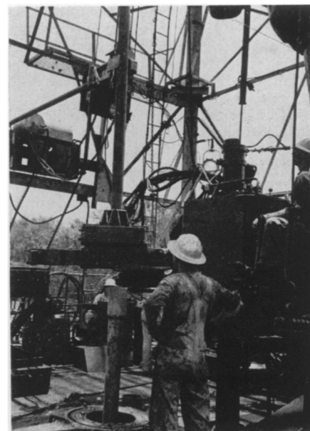
POWER TONGS —Rotary helper watches with hands on hips as the remote-control power tongs, controlled by the operator, "hand" a stand of five-inch drill pipe to lower pipe-racking arm. The pipe weighs nearly a ton.
