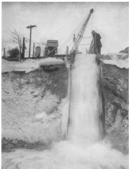
SOLVING WATER SHORTAGE —Here is shown the test pumping of one of the Ranney collectors. The test gave a yield of 9,800,000 gallons per day.
