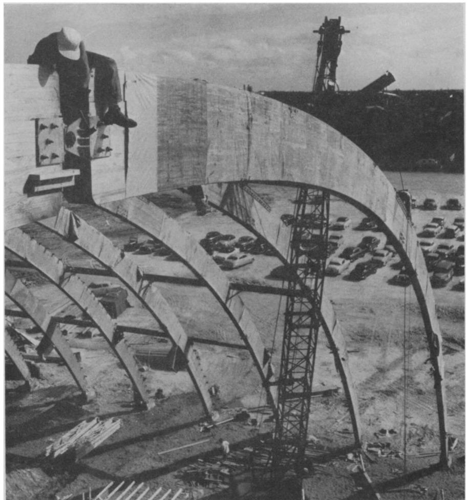
WOOD ARCHES —A workman fastens a shear plate to a wood arch made by gluing layers of wood together. This Florida sports arena has a 242.5-foot wood span, which would have been impossible in the U. S. 25 years ago. Today we have buildings with clear span timber structures of 250 feet and wood towers spanning to 300 feet.
