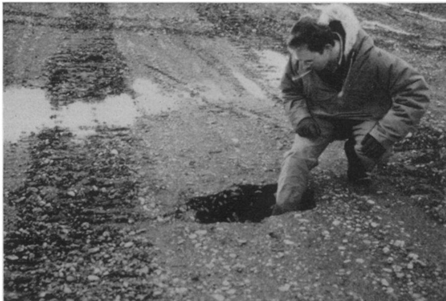
ALASKAN RUNWAY —The caving and irregular settling shown in this picture took place in a gravel fill over thawing ice wedges at Umiat, Alaska. This and many other construction problems are the result of disturbing nature's deep freeze locker.
