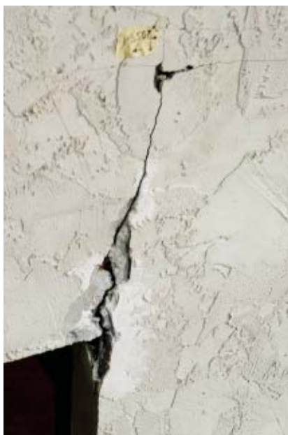
ALL CRACKED UP — Structural damage around the townhouse's garage door was severe, which is typical for such wide, unsupported spans.
